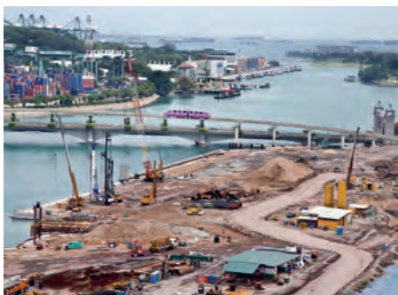
Top: At Sentosa Island, Singapore, we are treating excavated spoil, which is supplementing a dwindling supply of local sand.
