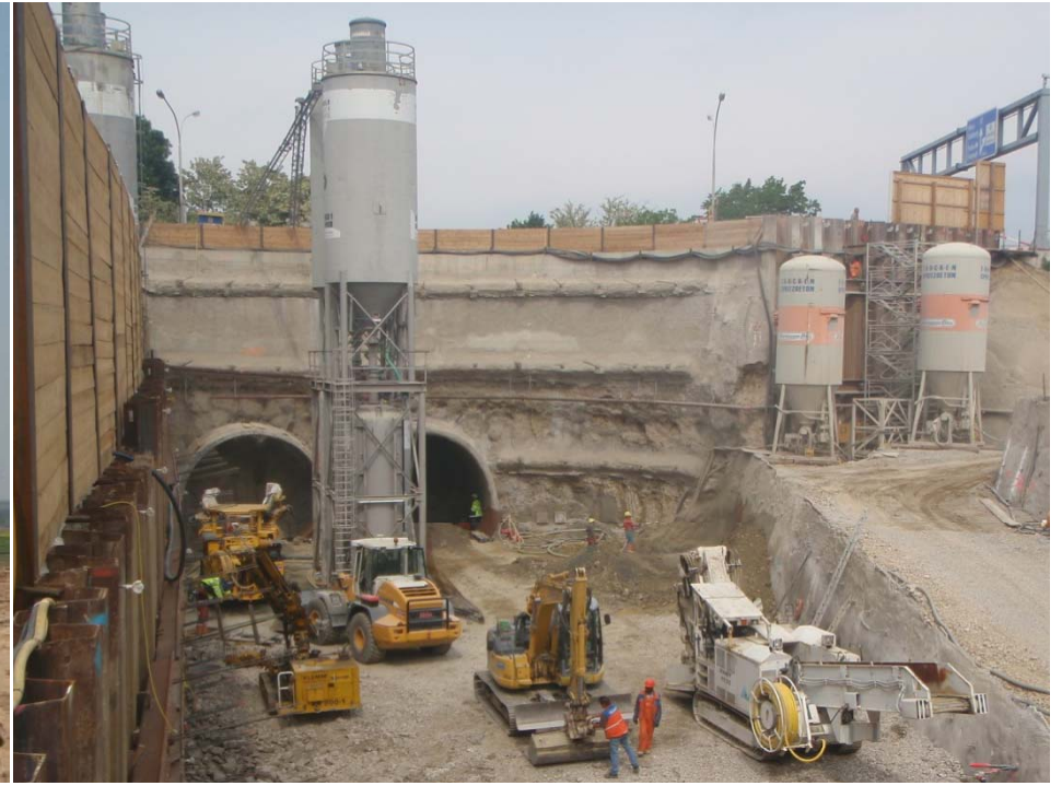
Western Europe New light underground tunnel, Linz, Austria Several products, including jet grouting and anchors
