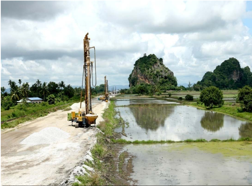
Ipoh to Padang Besar Railway, Malaysia Ground improvement for a new electrified double track
