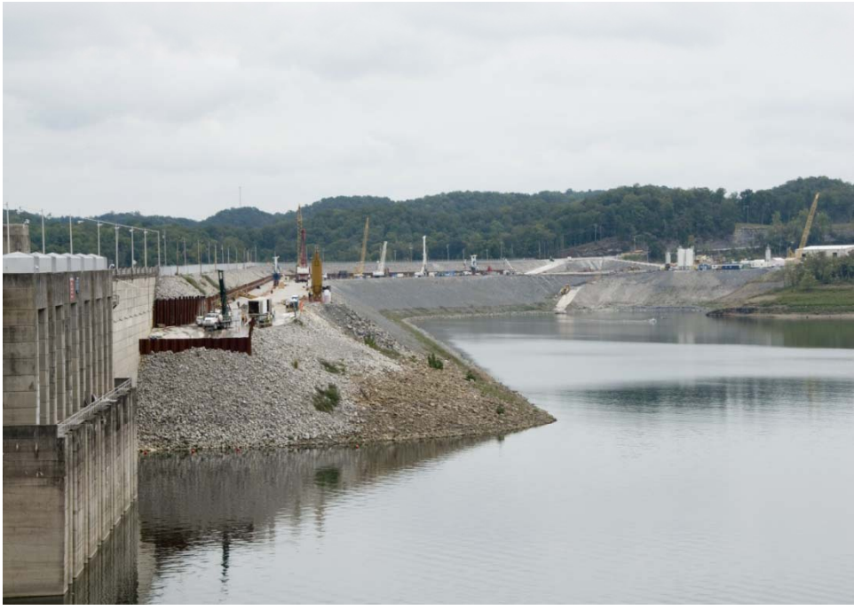
Remedial work at Wolf Creek Dam, Kentucky Drilling and grouting to cut off water seepage
