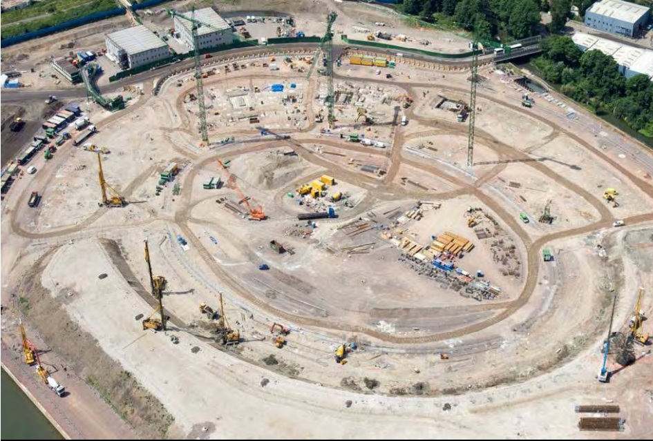
Foundations for Olympic Main Stadium, London Driven piles, CFA piles and Vibro concrete columns
