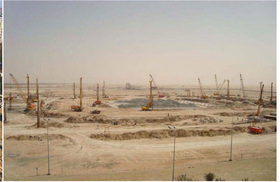
Middle East Khalifa Bin Zayed National Stadium, Abu Dhabi Piling and Ground improvement
