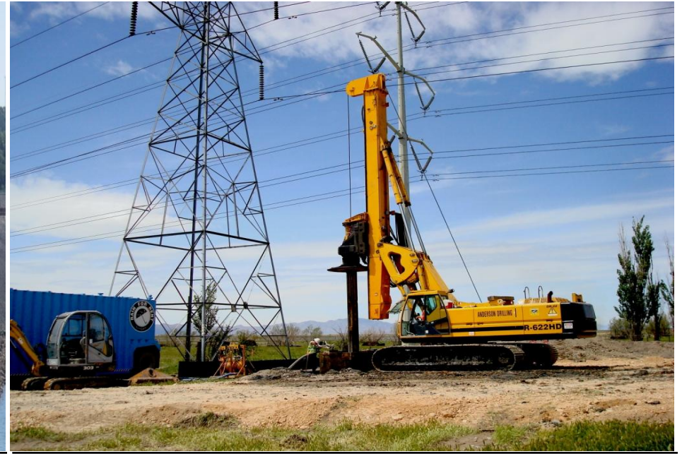
New power line near Salt Lake City Piling for the tower foundations
