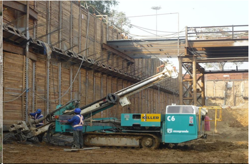
New Delhi Metro, India Removable anchors as part of retaining wall system
