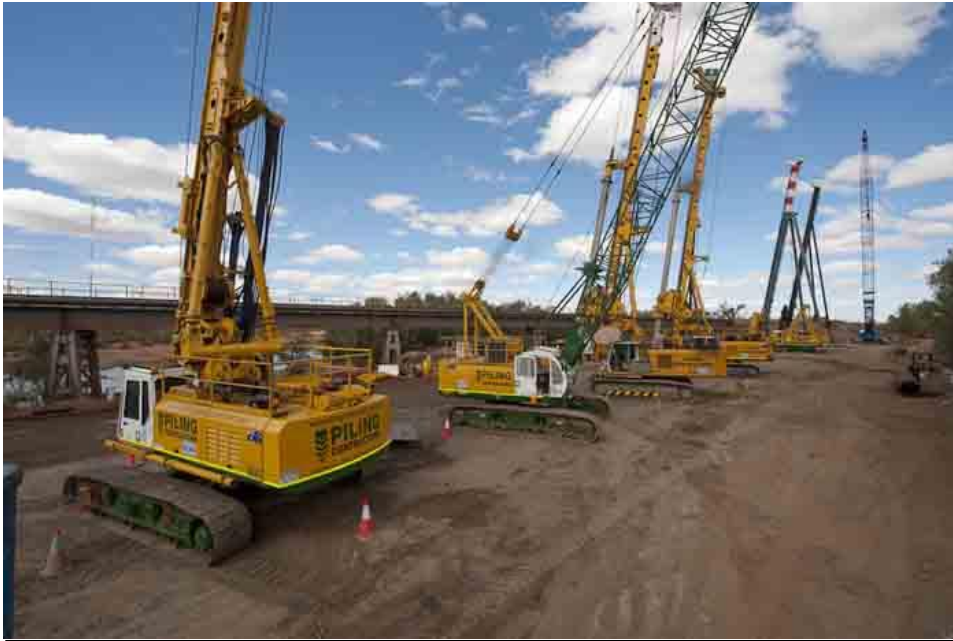
Rapid Growth Project, Western Australia Bored and driven piles for iron ore rail line
