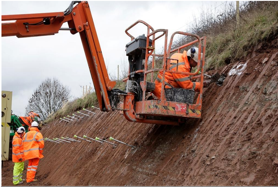
Widening of the M1 to four lanes, Nottinghamshire Soil nailing for stabilising embankments
